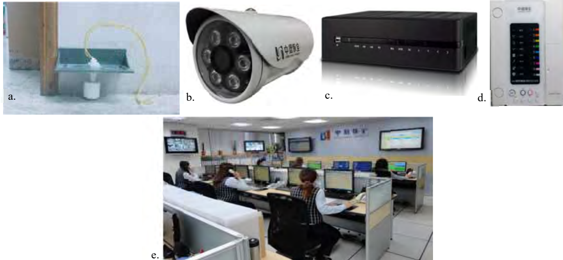
Figure 3. Smart technology system equipment for flood risk management: a) water level sensor, b) security reporting system, c) CCTV camera, d) security host, and e) the 24-hour control center
