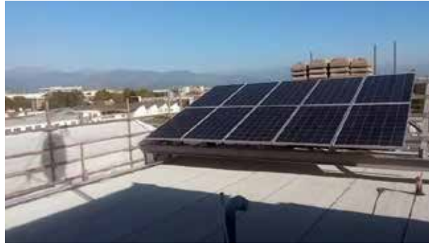
Figure 7 View of the roof, after the intervention. Source: Architettura senza Frontiere Piemonte.
