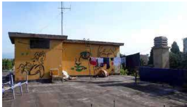
Figure 6 View of the roof, before the intervention. Source: Architettura senza Frontiere Piemonte.
