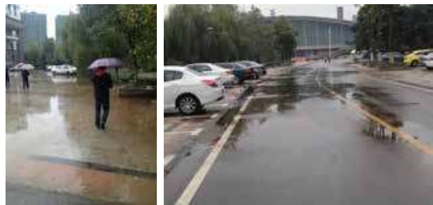
Figure 8 Water accumulation in impervious pavement
